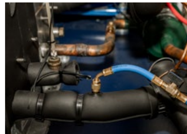
Connection hoses with ball valves for quick closing and opening of refrigerant flow.
