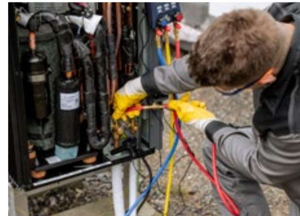
Easy to carry out maintenance work on heat pumps.
